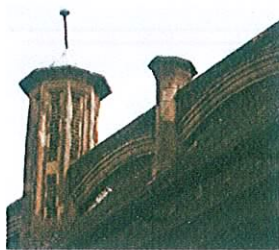
Overall view of the north aisle turrets showing decayed quoins and poor quality cement mortar repairs
