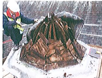
View showing decayed timberwork on turret
