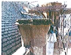
View showing decayed stone piers and copings turret
