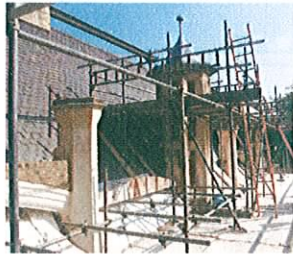
The decayed arch voussoirs (angled stones) were cut out and the arches reconstructed using new stone view showing temporary form-work
